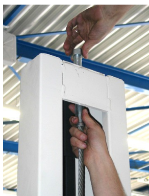
Figure 19: Cable run in column
